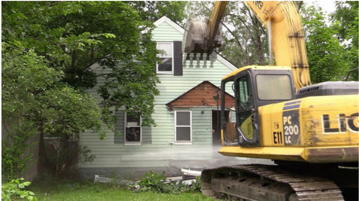
A backhoe starts the demolition of a foreclosed house on East 130th Street in Cleveland by the Cuyahoga Land Bank and Lightning Demolition and Excavating. (Dave Andersen/cleveland.com)
