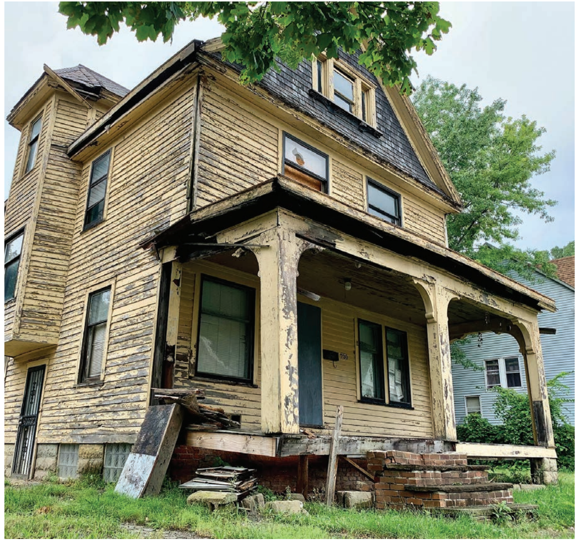
A dilapidated house sits empty on Cleveland's East Side. | MICHELLE JARBOE/CRAIN'S CLEVELAND BUSINESS
